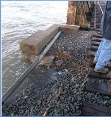
Railroads, highways and subways are all at risk from coastal flooding and salt water damage.
